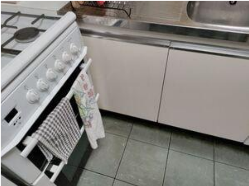
TMV behind panel in LHS sink unit
